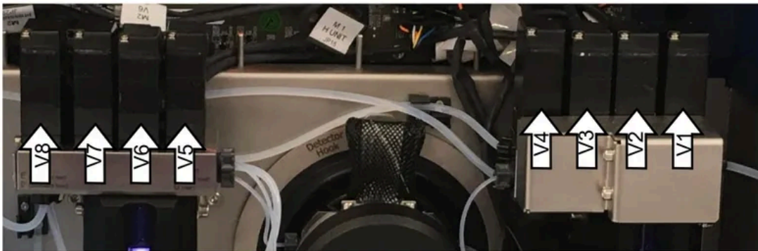
Fig. 11 Valves - Pump Manifolds
